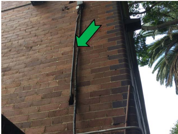
Photo 3. Exterior, north elevation, adjacent male toilets, insulation – non asbestos containing woven material.
