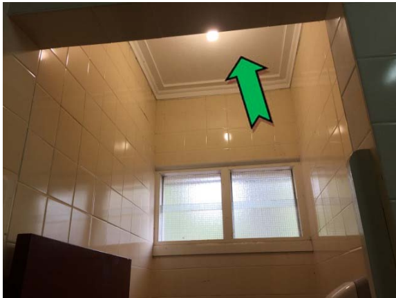
Photo 9. Interior, north bathroom, ceiling – non asbestos-containing fibre cement sheeting.
