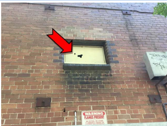
Photo 5. Exterior, west elevation, infill panels at height – suspected asbestos-containing fibre cement sheeting.
