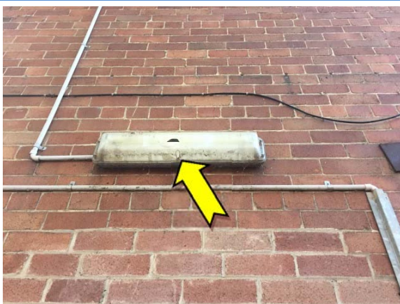
Photo 11. Exterior, single tube fluorescent light fitting – suspected PCB-containing capacitor.
