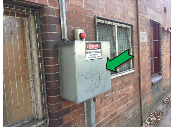
Photo 2. Exterior, ground level, north-west elevation, to wall, electrical switchboard – suspected non asbestos-containing bituminous material.
