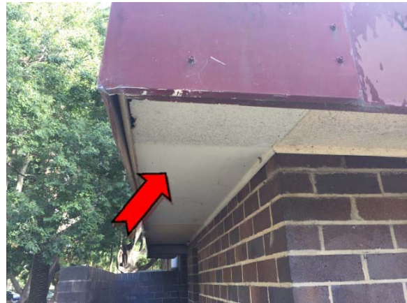
Photo 4. Exterior, south-west corner to female toilets, eaves – asbestos-containing fibre cement sheeting.
