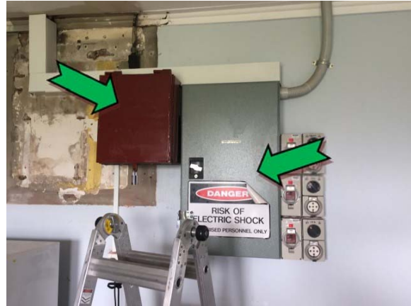
Photo 8. Interior, office, west wall, electrical boards – suspected non asbestos-containing electrical backing boards.
