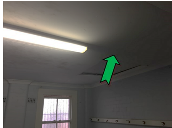
Photo 10. Interior change room one and two, ceiling – assumed non asbestos-containing fibre cement sheeting.
