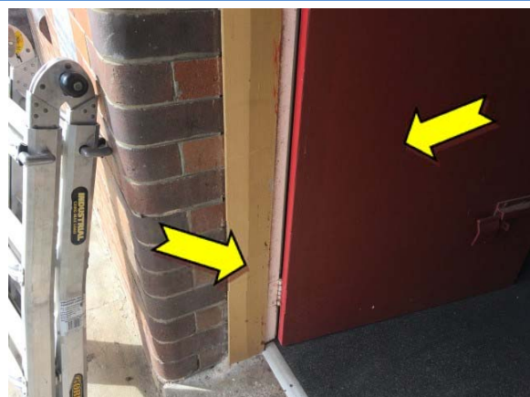
Photo 12. Exterior, door and door frames – suspected lead-containing red and yellow coloured upper paint systems.
